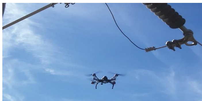
Figure 5.6: Dasmarias-Las Pinas 230 kV Line Inspection of parallel groove clamps and insulators for potential deterioration
